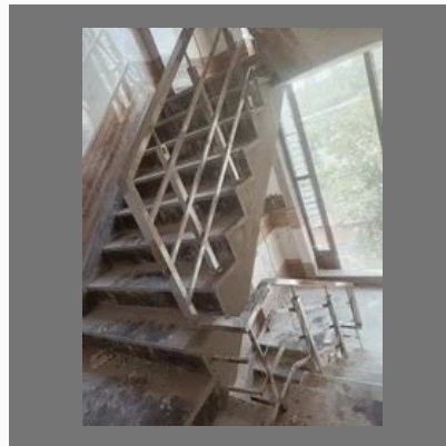
Stainless Steel Staircase Railing
